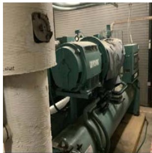
Water Cooled Chillers Serving CSS
