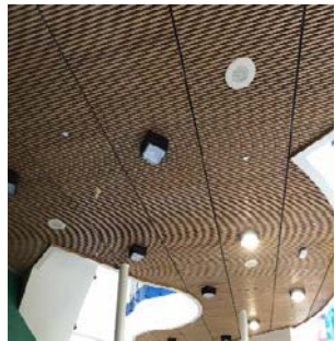
Ceiling Mounted MV and LED Fixtures
