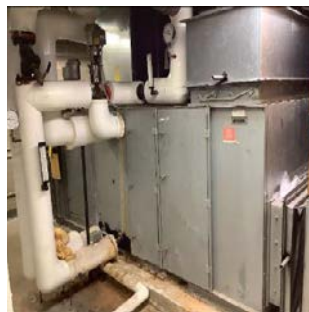
Air Handling Unit
