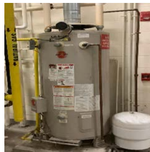
DHW Heater in ECC Section
