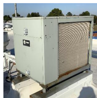
Condensing Unit Serving Kitchen MUA
