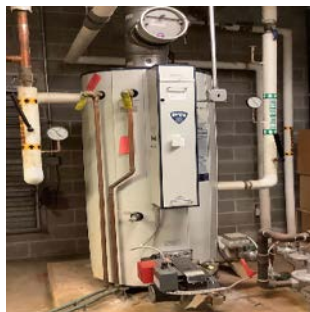
DHW Heater in CSS Section
