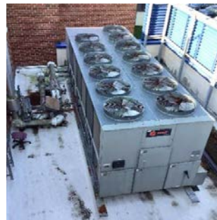
Air Cooled Chiller Serving ECC
