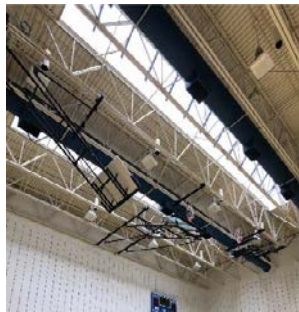
Gym Lighting Fixtures
