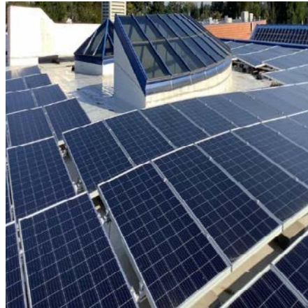
Rooftop Solar Array
